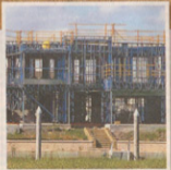
Harbour Quays is the site for this new home built with a locally made steel frame
